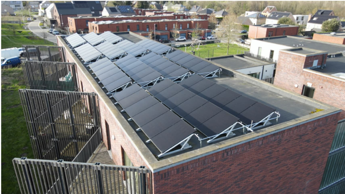
Figure 28: Overview of PVT installation
