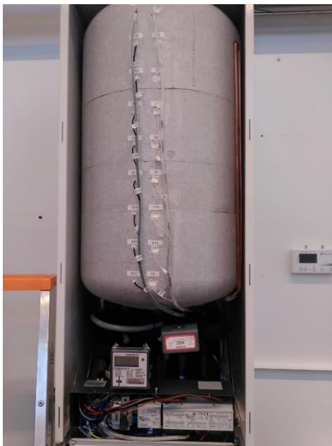
Figure 30: District heating satellite unit
