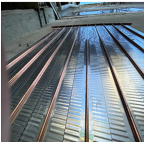
Figure 7: Active heating and cooling layer design applied to the outside of the existing building facade
