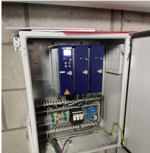
Figure 31: Phase angle controller for P2H control via BEMS
