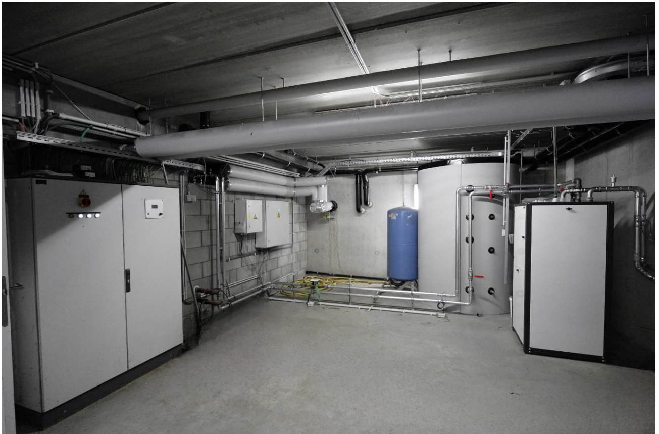
Figure 26: Overview of heat pump with high temperature storage and control cabinets
