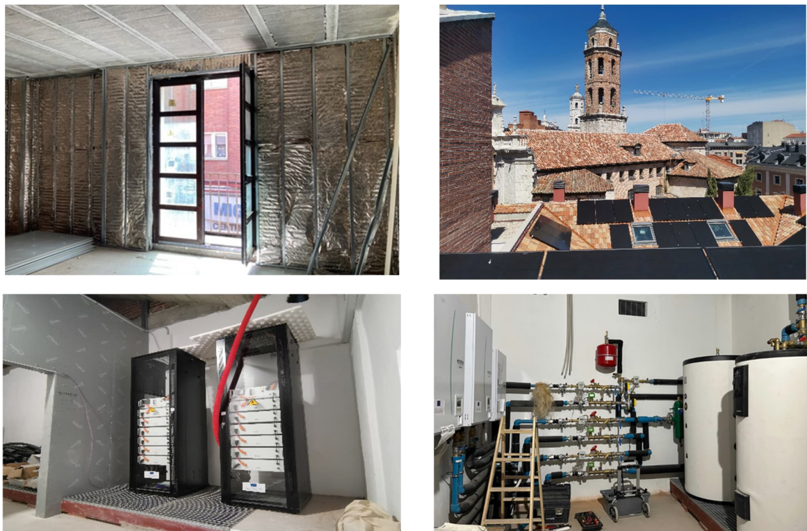
Figure 1: Key components of the Spanish Demo energy system: high performance thin insulation (upper left), PV installation (upper right), battery energy storage (lower left) and air-source heat pumps with storage tanks (lower right)
