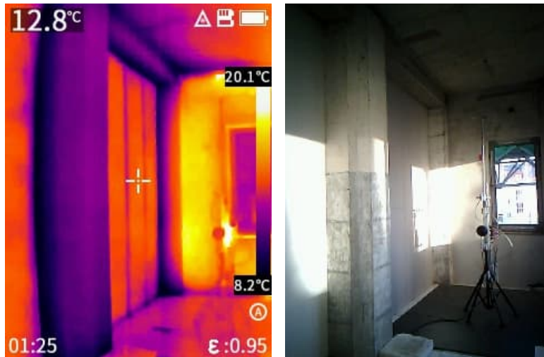
Figure 39: Thermographic image (left) of the thermally activated facade and opposite inside wall seen from the inside of the demo room and visible spectrum reference image (right)
