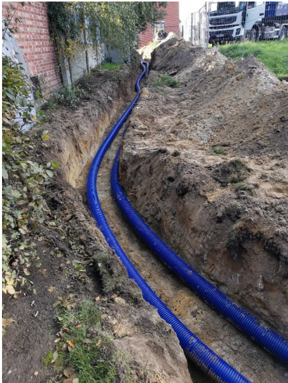
Figure 29: Solar heat transport pipes to boiler room
