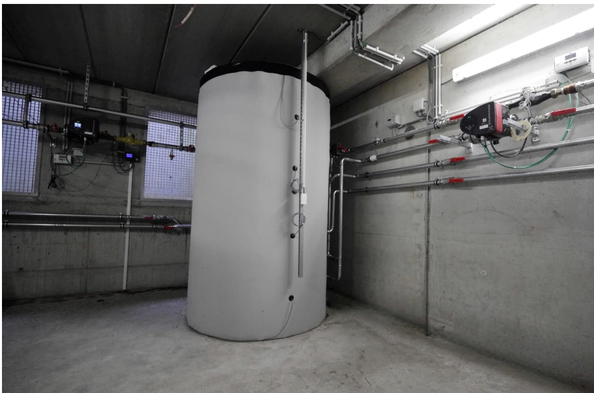
Figure 25: Low-temperature storage tank which connects HP, PVT and BTES
