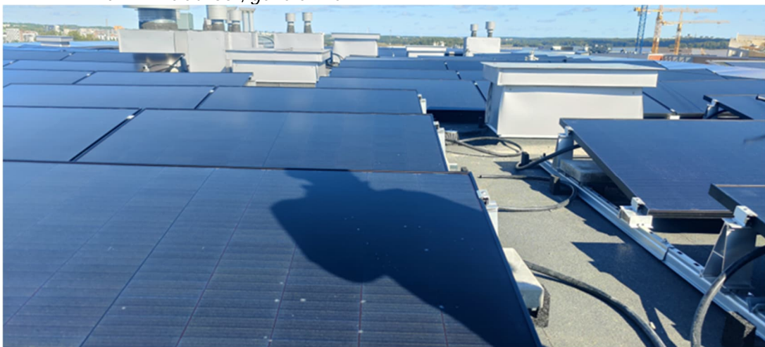
a. PVTs at roof, details
